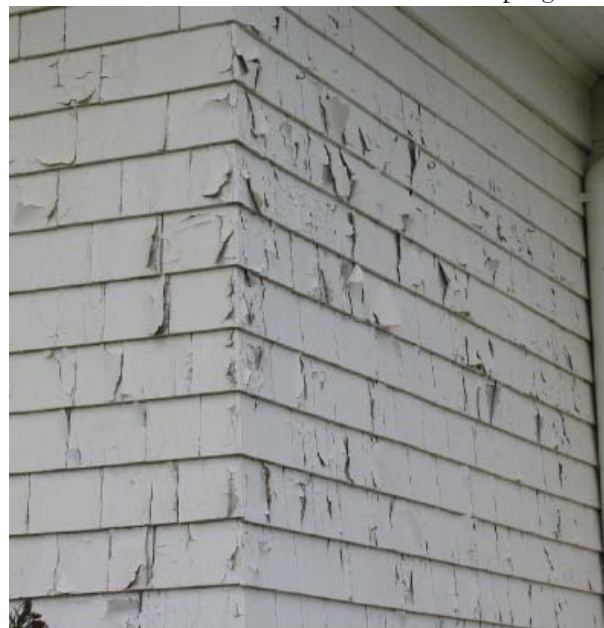
Fig. 36 : Much of the paint has detached from the shingle siding.
