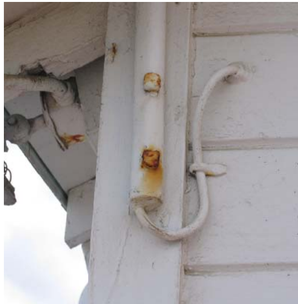
Fig. 40 : Corroded ferrous metal hardware is embedded in the shingles
