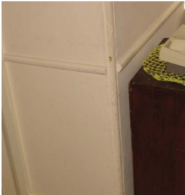
Fig. 59 :Flat plaster wall and corner bead at the interior of the Officer in Charge Quarters.
