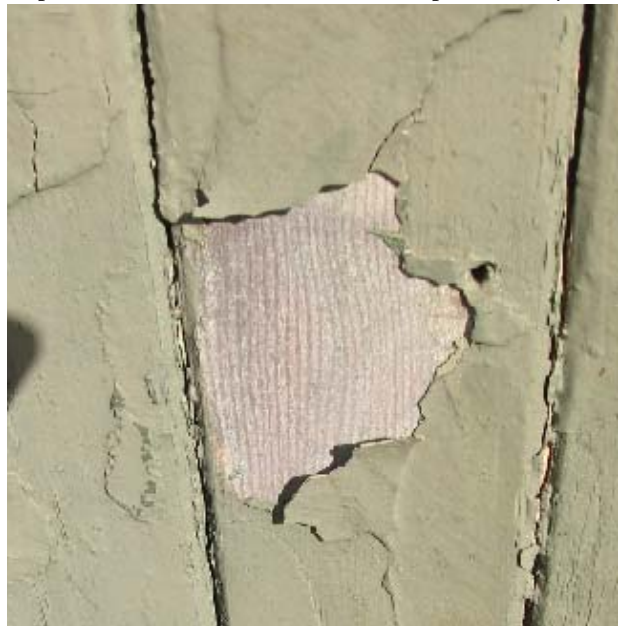
Fig. 46: Paint failure on the doors of the Shop & Garage.
