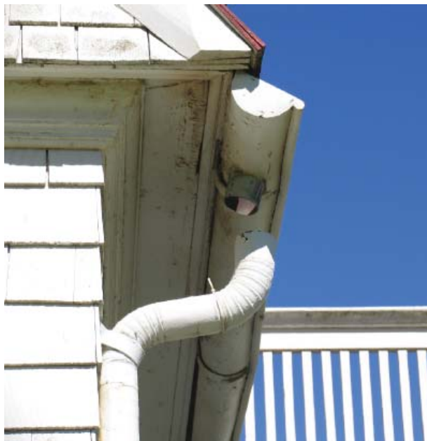
Fig. 29 : Disconnected drain spout at the Officer in Charge Quarters.
