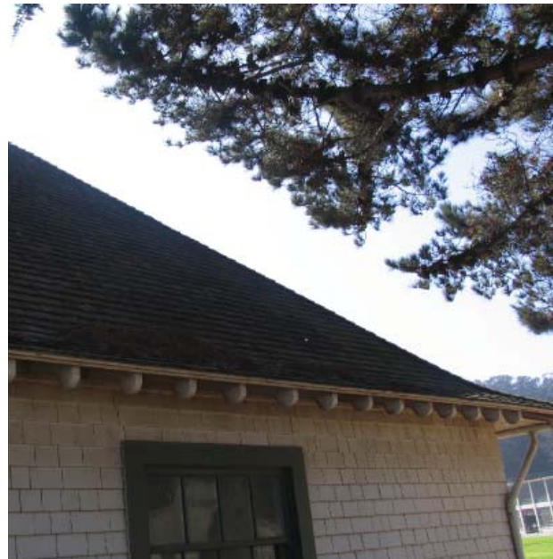
Fig. 56: Overhanging tree limb at the 1890 Boathouse.
