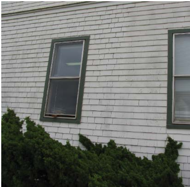
Fig. 55: Vegetation at the south wall of the Main Boathouse.
