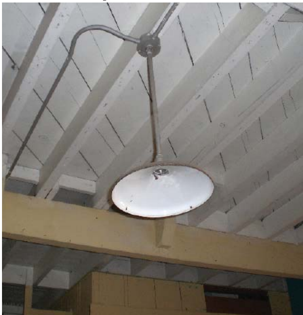
Fig. 71 : Historic pendant light fixture at the Shop & Garage.
