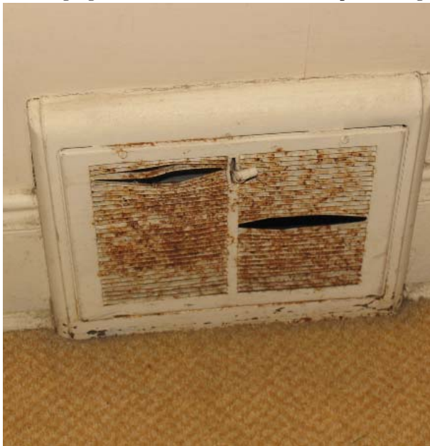
Fig. 73 :Heater vents at the Officer in Charge Quarters.
