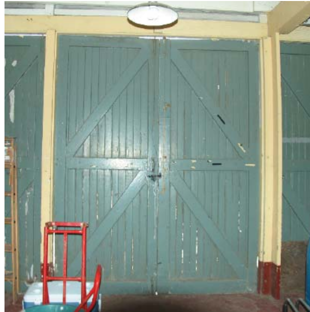
Fig. 68 : The doors at the Shop & Garage appear to be in fair condition.
