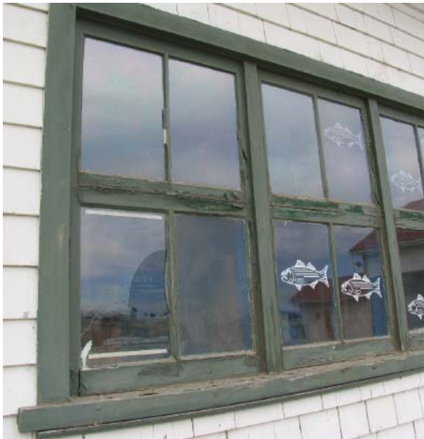
Fig. 33 : The exterior paint is deteriorating on the windows, as is the glazing compound.
