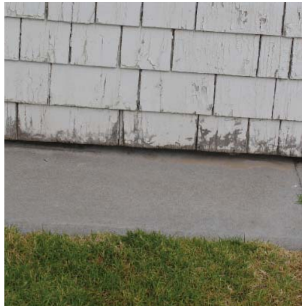
Fig. 34: Improper drainage at grade has lead to shingle deterioration.
