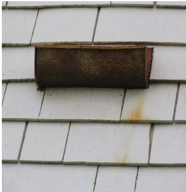
Fig. 39 : Rust stains are evident in the shingled areas.
