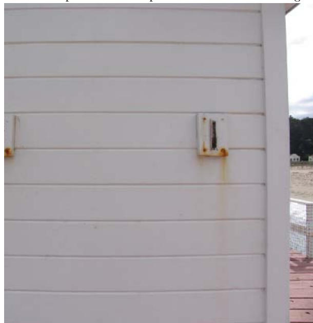
Fig. 43: Corrosion staining from embedded hardware at the Buoy Shack
