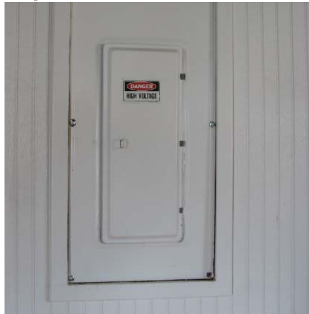
Fig. 72 : Electrical box at the Buoy Shack.
